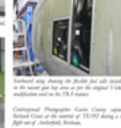
Overhaul work showing the fuselage just cells installed in the main gun bay area as per the original 1945 repair manual and on the TE392 fuselage.
